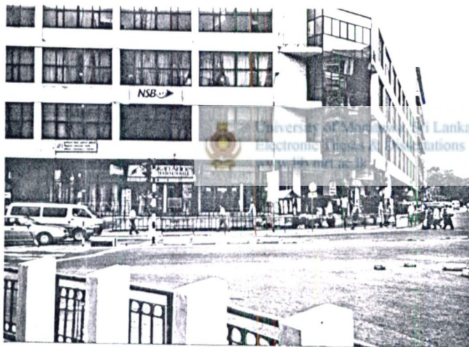
Fig. 113 Wrong Connection between elements
