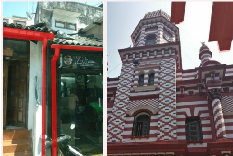
Fig. 4: Rainwater discharge Source: author
