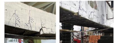
Debonding & Cover delamination
