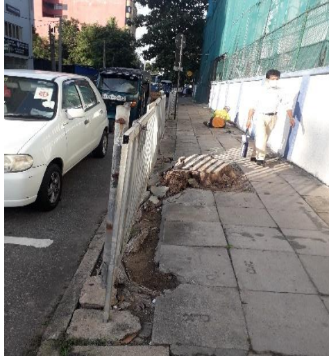
Figure 4:24: Obstruction of tree stump on pavement Source – Author
