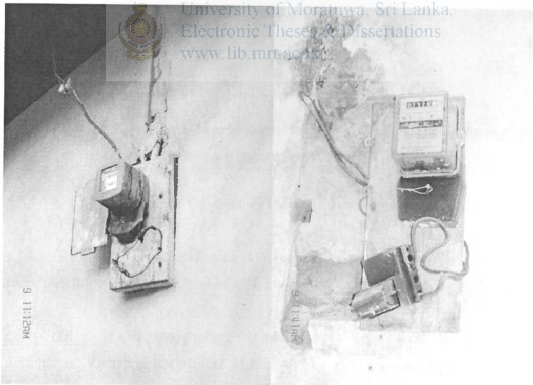
Poor maintenance of consumers' energy meters increase revenue losses
