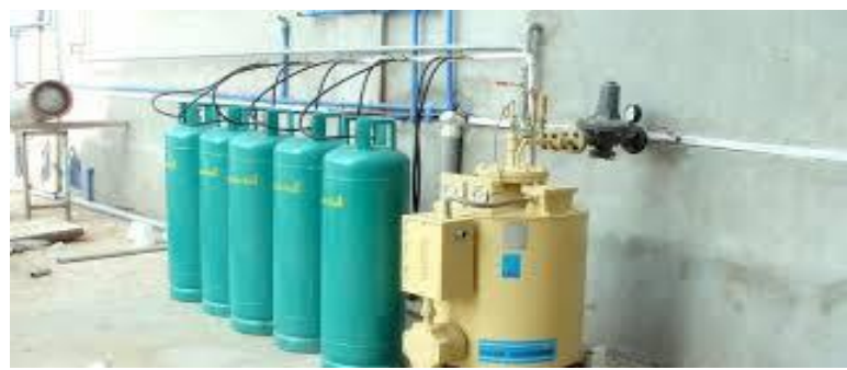
Figure 14: Liquid withdrawal manifold with Vaporizer
