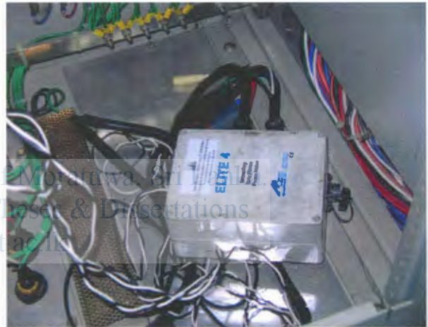
4.1 (b) Analyzer connected for 132kV measurements
