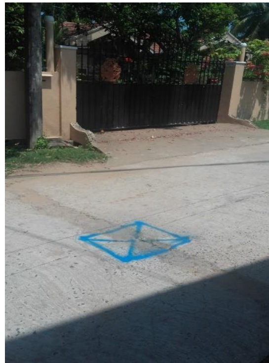
Figure 5.18 : Marked detected leak point
