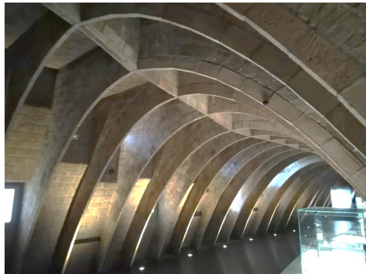
Figure 2.14: The support structure for the roof terrace at the attic of Casa Milla, Barcelona.
