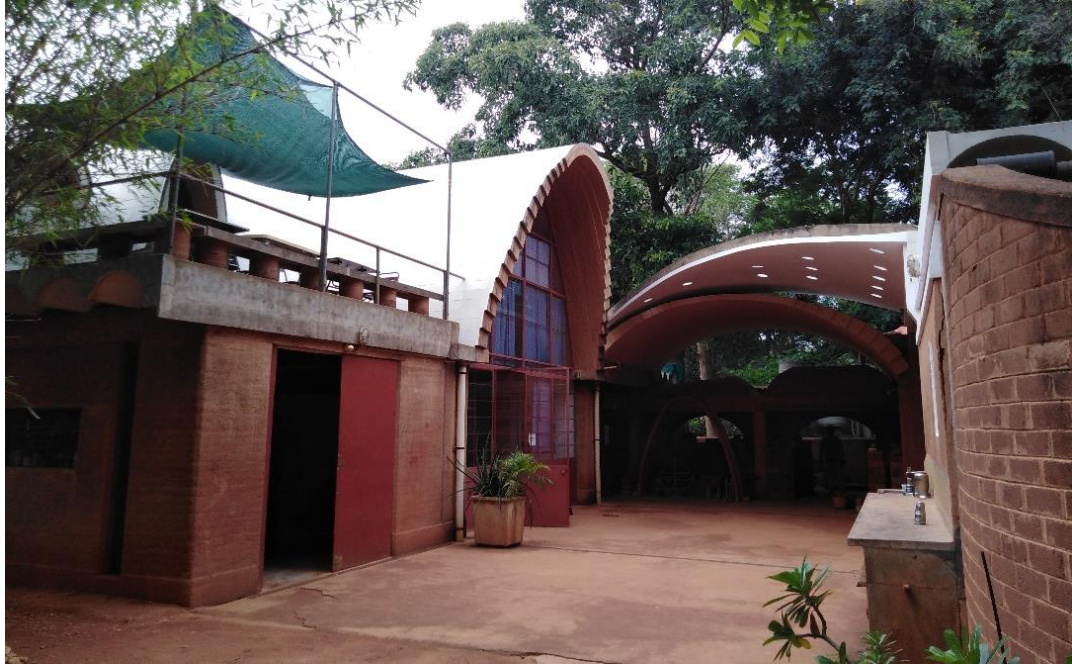
Figure 2.20: Vaults and thin shells at Auroville Earth Institute (AVEI), Tamil Nadu India.
