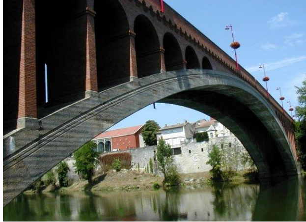
Figure 2.21: Pont de la Liberation Bridge in France, constructed of unreinforced concrete. Source: Structurae.net/ Photographer: Jacques Mossot.
