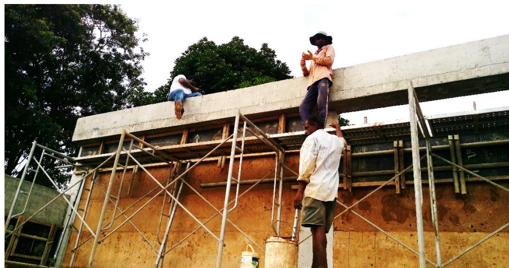
Figure 115: a)-Step one; Formwork (F) assembling for 16'-0" length and 4'-0" height. b) - Step two; bottom formwork dissembling and assembling the top formwork. 02 nos. of labour (L) required for formwork assembling and 02 labour (L) was required for mixing and pouring the MC mix.
