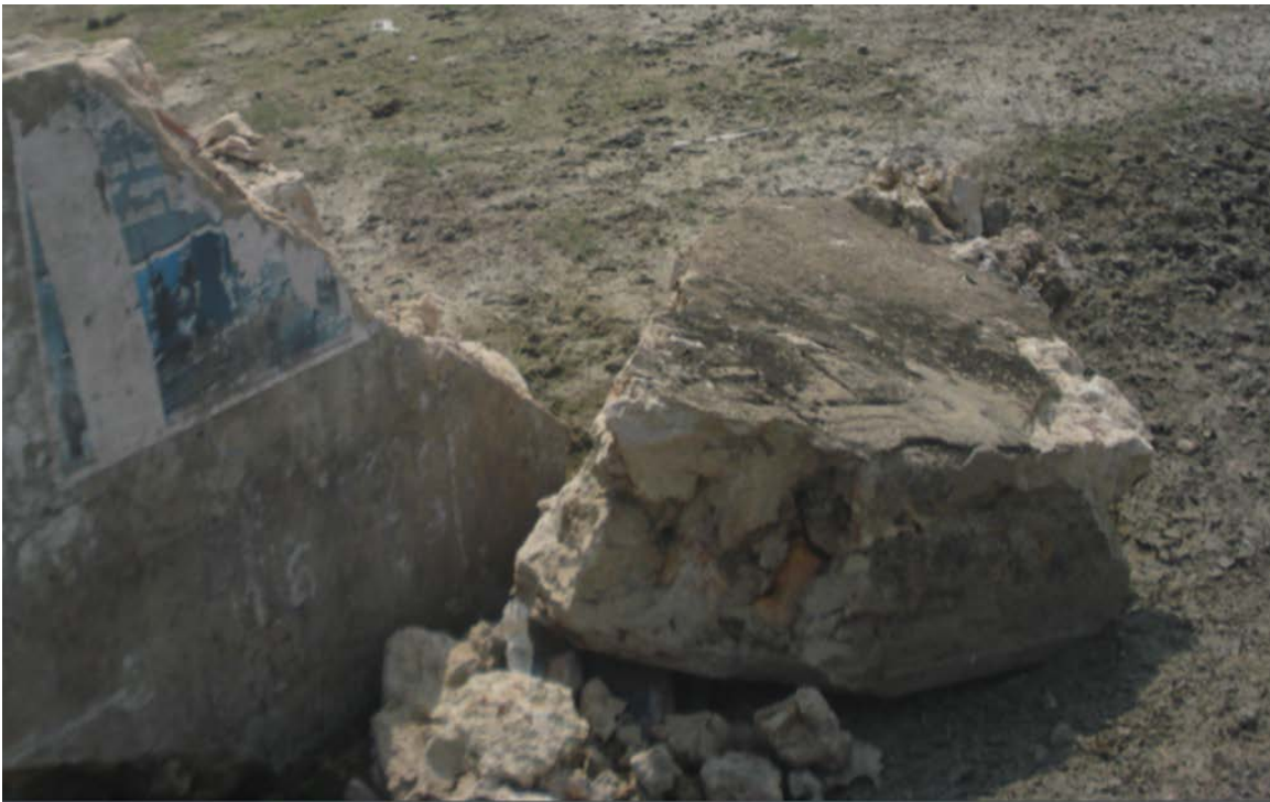
Figure A15.2: Concrete Debris
