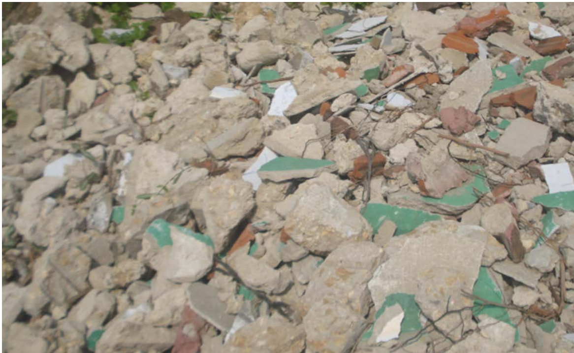
Figure A15.4: Cement Plaster Debris
