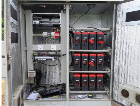
Figure 7.6 : Existing VRLA AGM 300Ah Battery Bank at Karandana Mobitel Site
