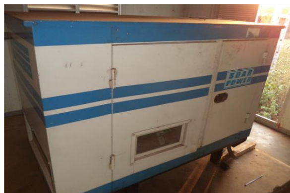
Figure 7.1 : Installed 8kV Generator at Welimuwapotana Dialog Site
