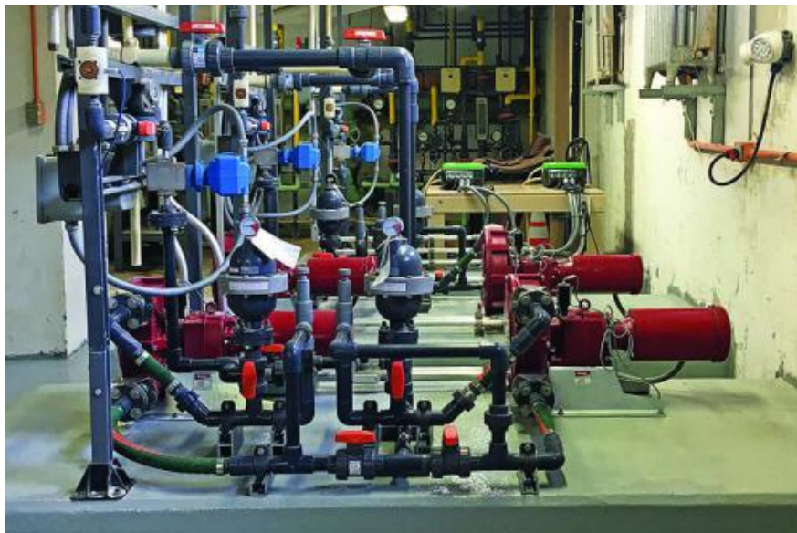
Figure 4.9: The Omohundro plant alum feed system, showing the feed pumps, pulsation dampeners, flow meters, carrier water system, isolation valves, and pressure relief valves
