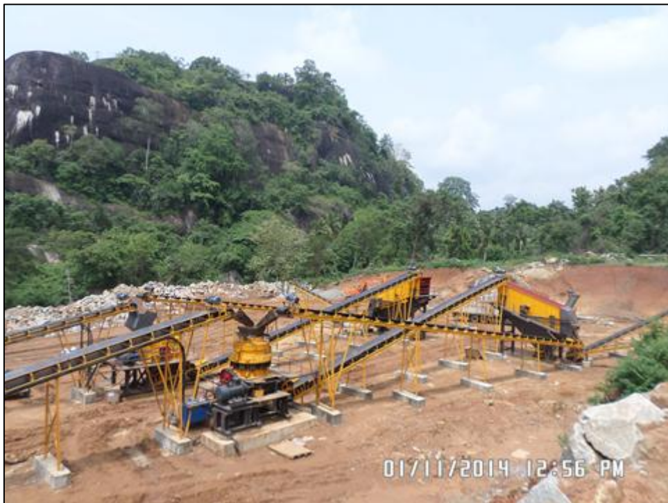
Figure 24: Second Stage Crushing in Proposed Crusher Plant
