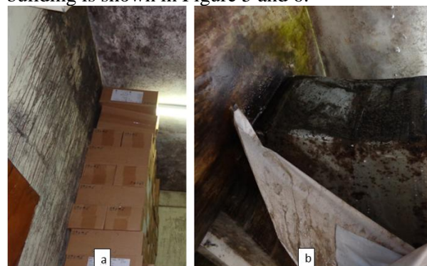
Figure 5: Severe mould growth (a) ICU store room S2 at second floor (b) A duct in S5 at second floor
