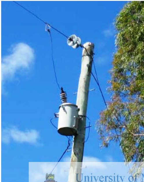
Figure 2.3 SWER distribution transformer.
