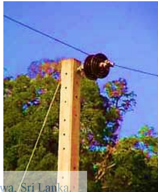
Figure 2.4 SWER line connected to pole
