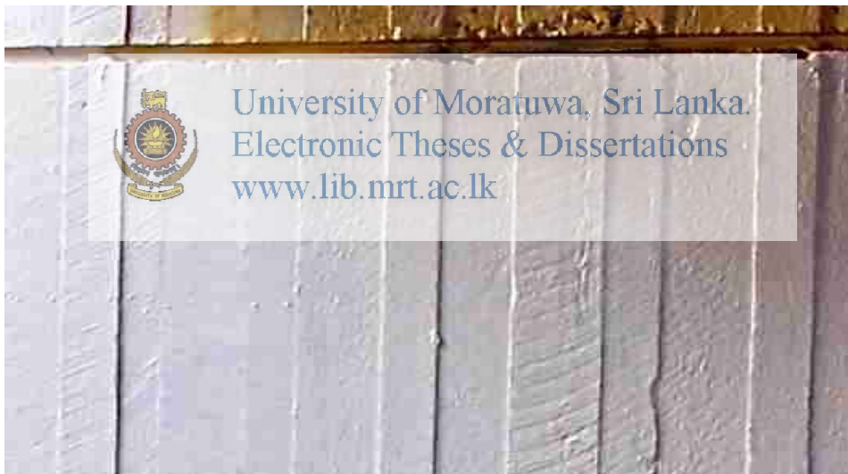
Figure 04: Poor finish in conventional type formwork
