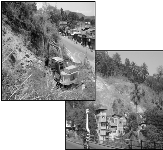
Figure 4 Landslide mitigation programme in 2010
