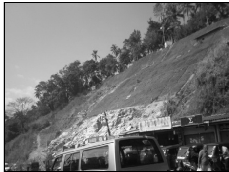
Figure 5 Current situation of Landslide mitigation by 2012
