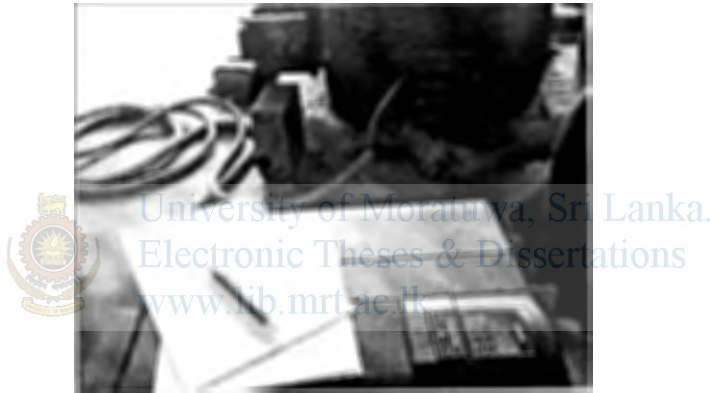
Fig-4.5: Perform Motor Identification Routine of a VSD for 11kW WRIM
