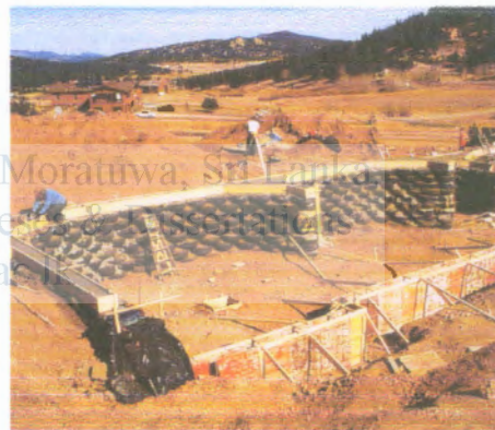
Fig 02: Concretebond beam served as a surface on which to connect the tire walls and wood roof framing.
